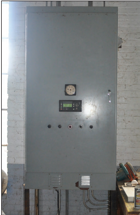
A. Circa 2000 Control Panel Boxes
