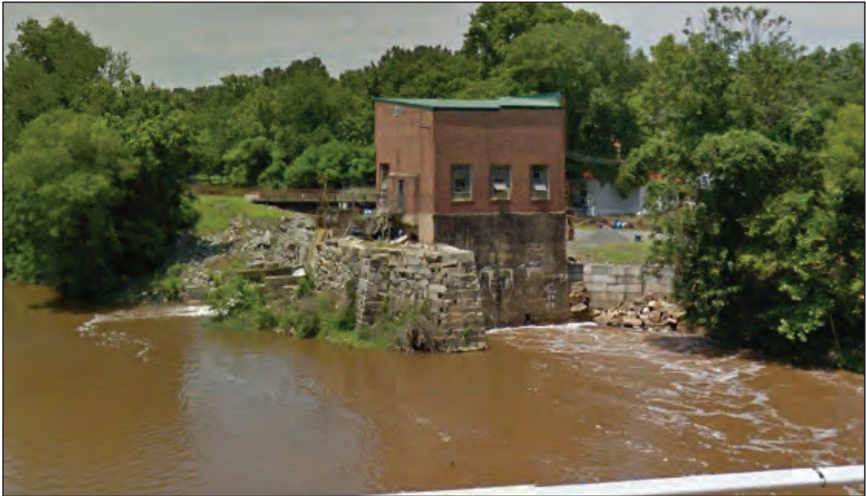
A. View of Lockville Powerhouse Looking North from Old US I Bridge Over the Deep River Source: Google Earth, 2017
