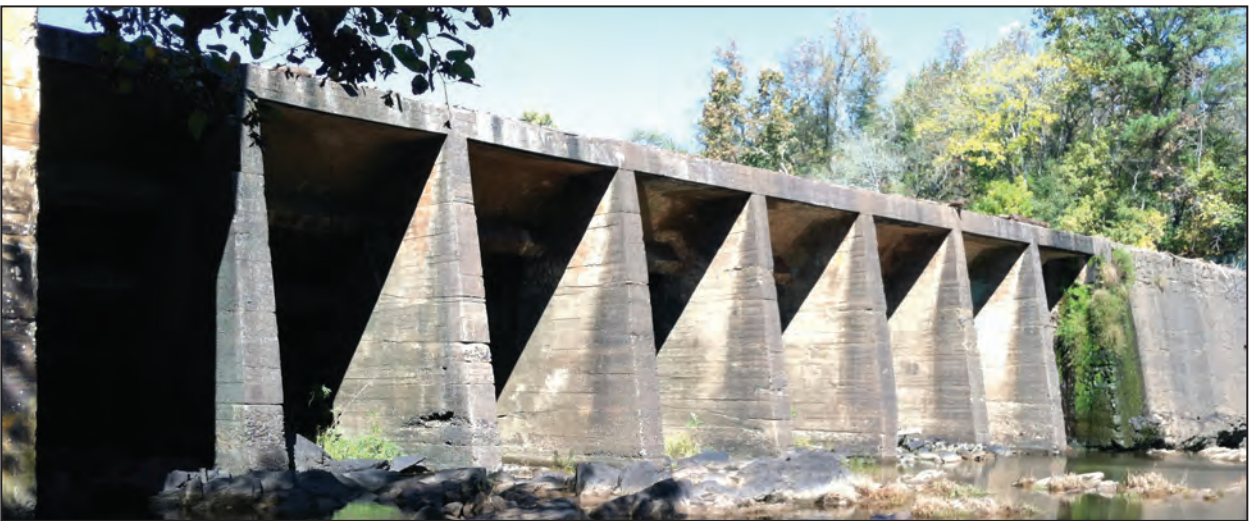
B. Downstream Side of Dam Looking Northeast from South of Powerhouse Photograph by Chris Flowers
